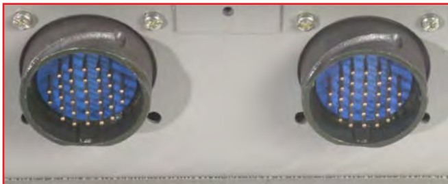
3 CT Cable Inputs (24 Units Total)
